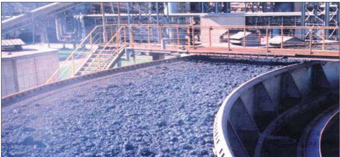
Figure 5.7 Circle Cooler of the sinter plant (Voest Alpine Industrianlagenbau [VAI] ,2008).
