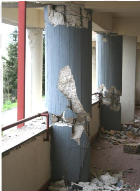
Figure 2.2: Damages to The Moment Frame That Has Been Precast.
