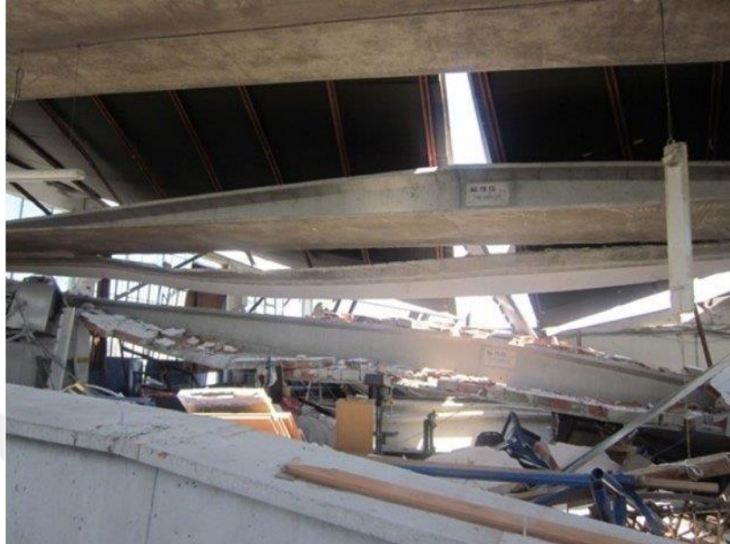
Figure 2.1: Collapse of Precast Building.
