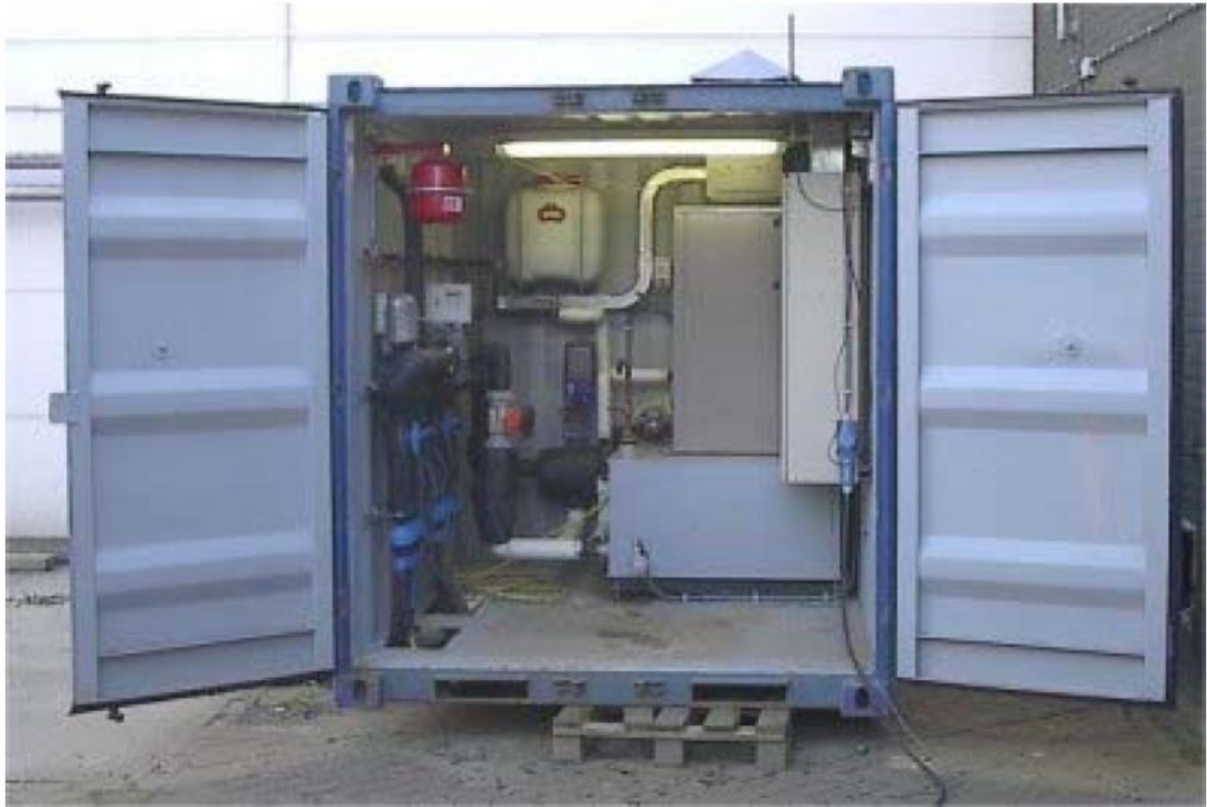
Figure A.5 : Dutch thermal response test rig with heating and cooling mode. Photo: Groenholland.
