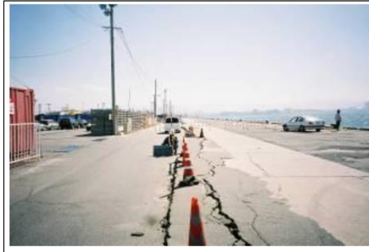
Figure 2.21 Liquefaction behind quay wall (Hamamoto et al., 2016)
