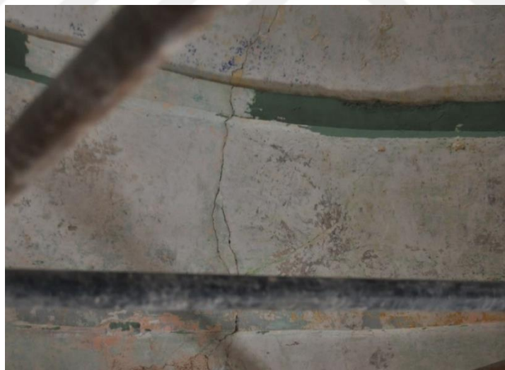
(b) Interior crack on the octagonal drum
