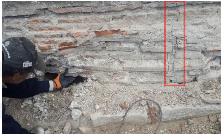
(a) Exterior crack on the octagonal drum
