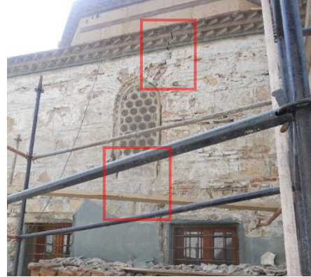
(b) Cracks on the east façade
