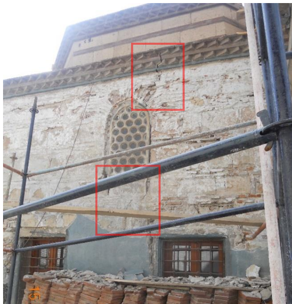
(a) Vertical crack on the East façade
