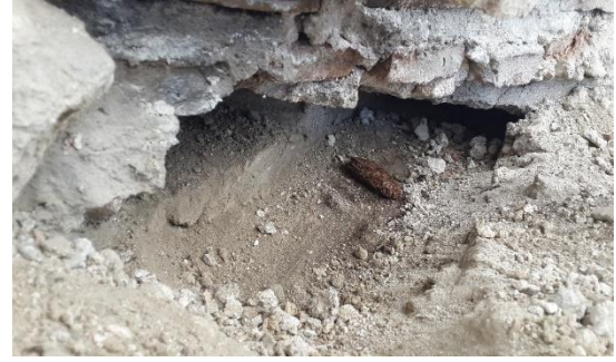
(b) Loss of wooden beam
