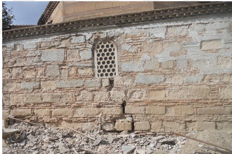
(a) Vertical cracks
