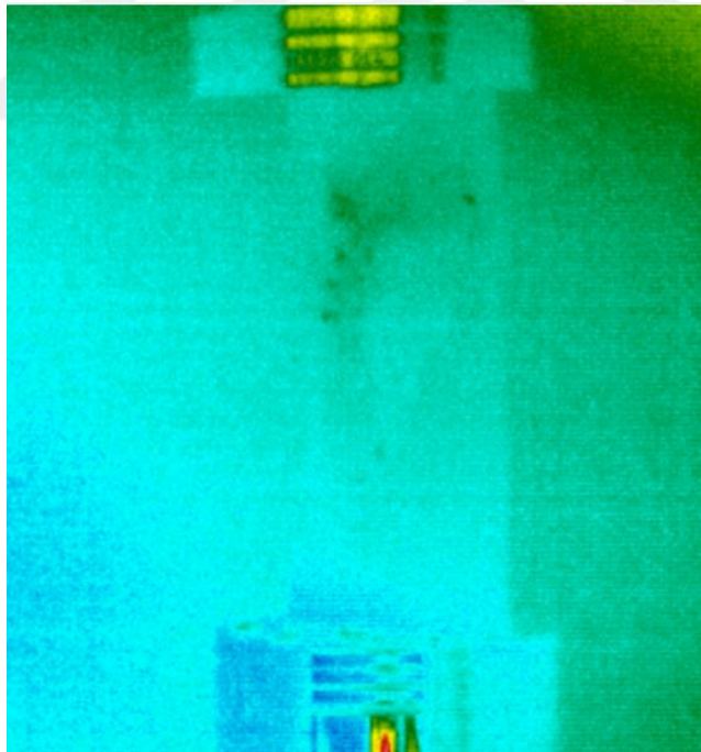
Figure B.2. Failure plane detection of the 75A-4 sample by the thermal camera
