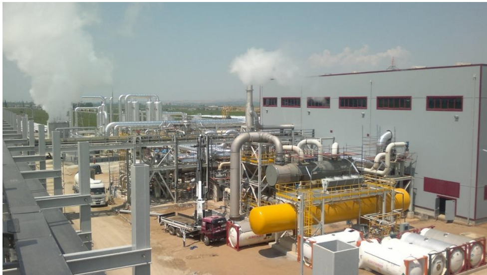
Figure 4.6 A Geothermal Power in the study area (Personal archive, 2019)
