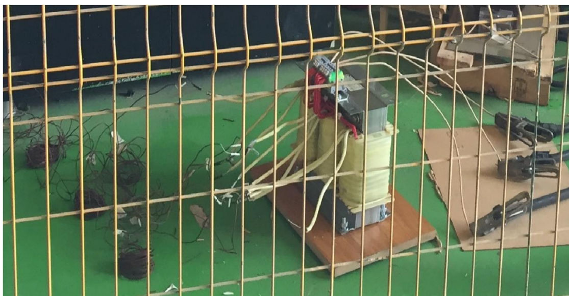
Figure 3.17 Cable Connections of 3 kVA transformer
