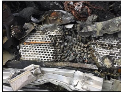
Figure 1.2: Lithium-ION Batteries Explosion in EV's [2].
