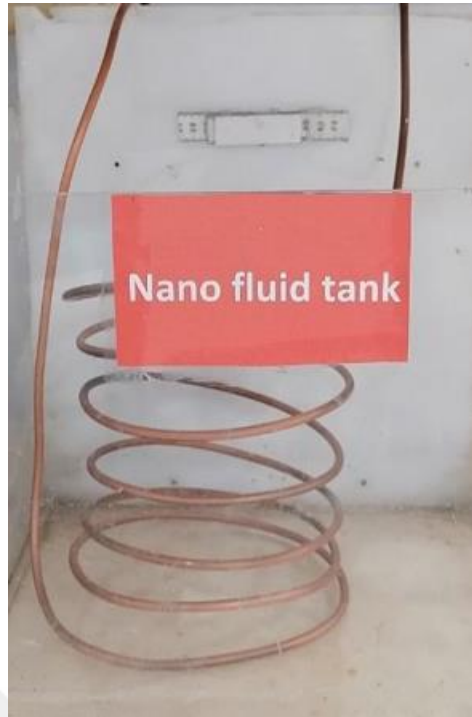
Figure 3.3: Cooling System Inside the Nano-Fluids Tank.
