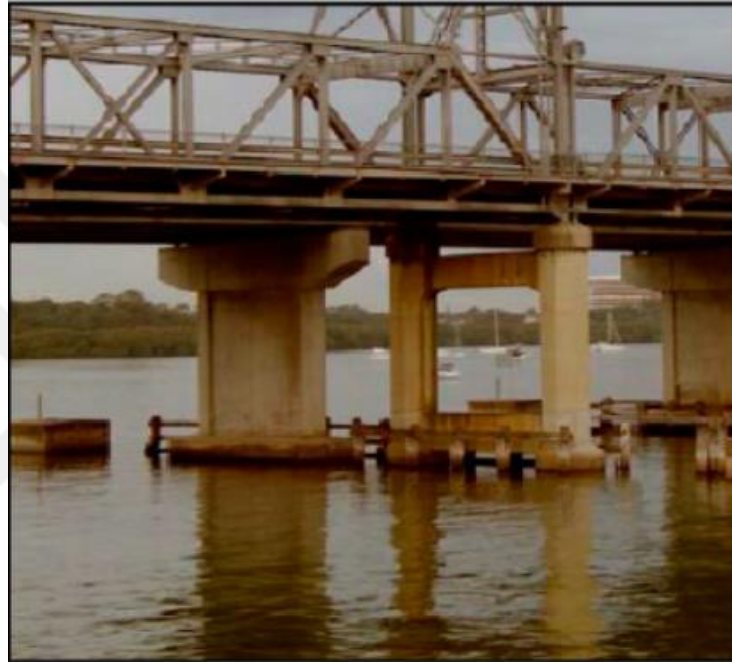
Figure 1-2: A case of scour in the foundation of Ryde Bridge in Sydney, Australia [7].
