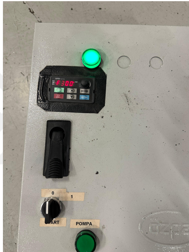
Figure 3.9. Electric motor controller.
