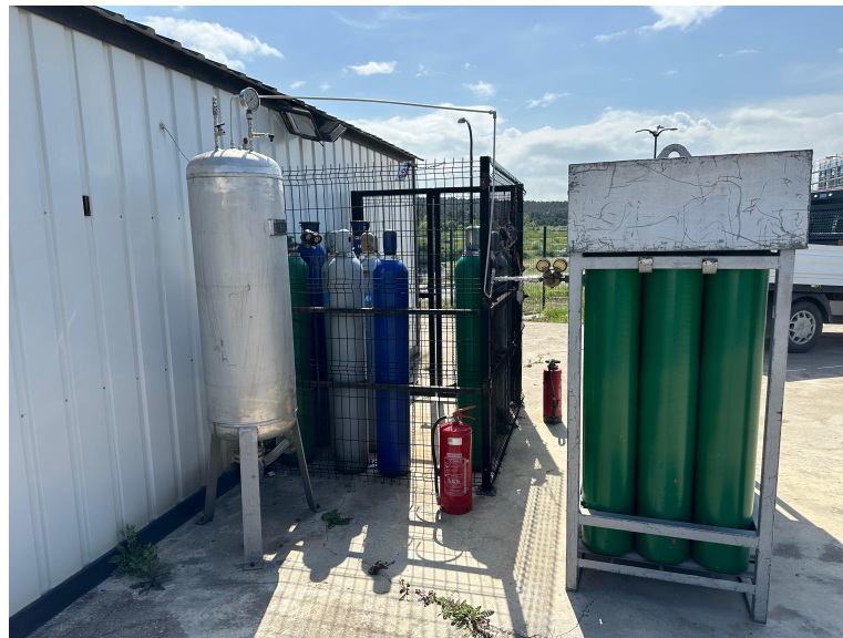
Figure 2.16. Water tank and nitrogen manifold used for pressurization at GÖRTEM Test Center.
