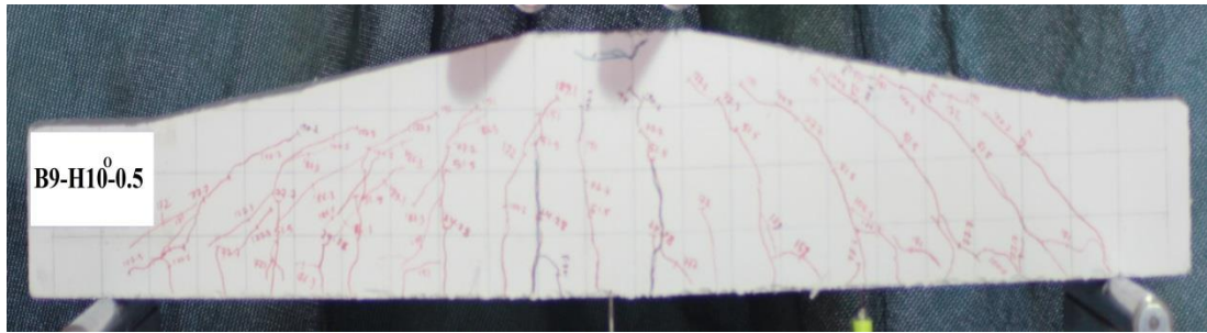
Figure 4.19 Flexural Failure Mode
