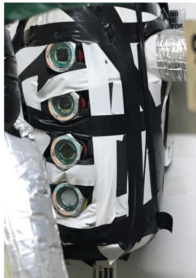
Figure 8.11 Liquid refrigerant and oil accumulation in the liquid-vapor separator (Personal archive, 2020)
