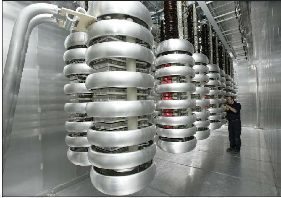
Figure 3. 22 HVDC power facility with VSC technology manufactured by ABB company [91], [119].
