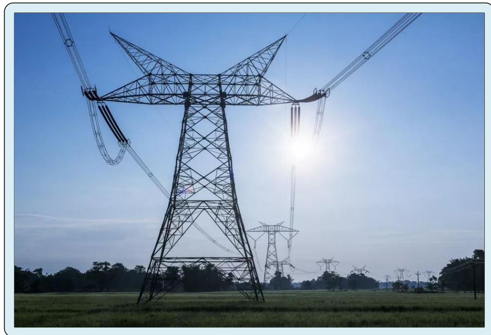
Figure 3. 33 A particular instance study of HVDC technology's overhead electrical power transmission lines [138].
