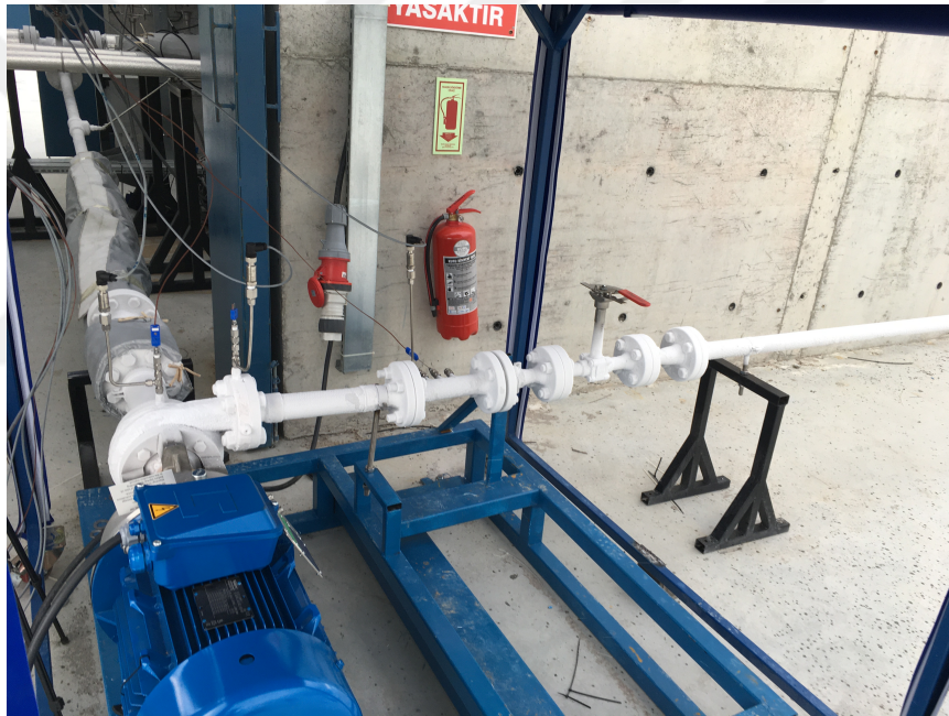
Figure 6.19: Condensation during cryogenic testing.
